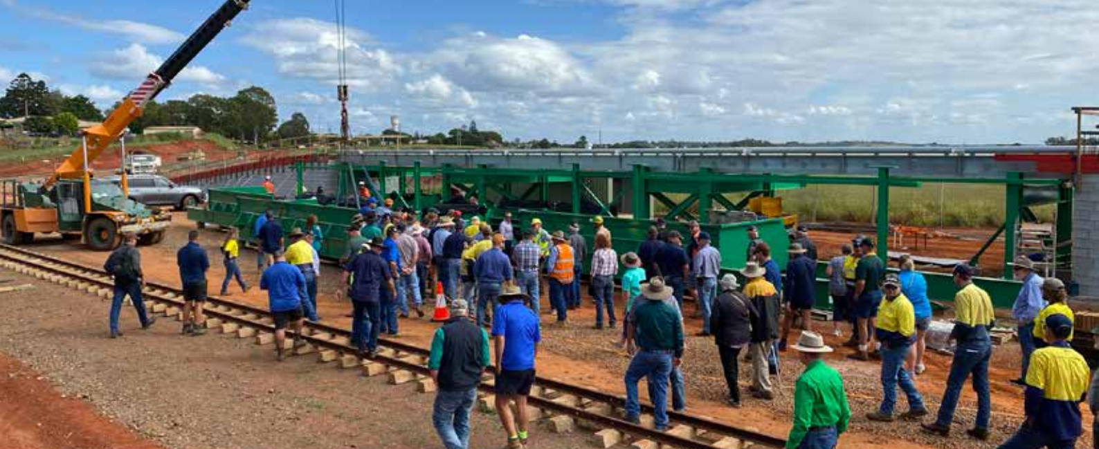
CANEGROWERS members visit the site of a transloader, being built to transfer Maryborough district cane to rail transport to access the Isis Central Mill after the closure of the Maryborough Mill
